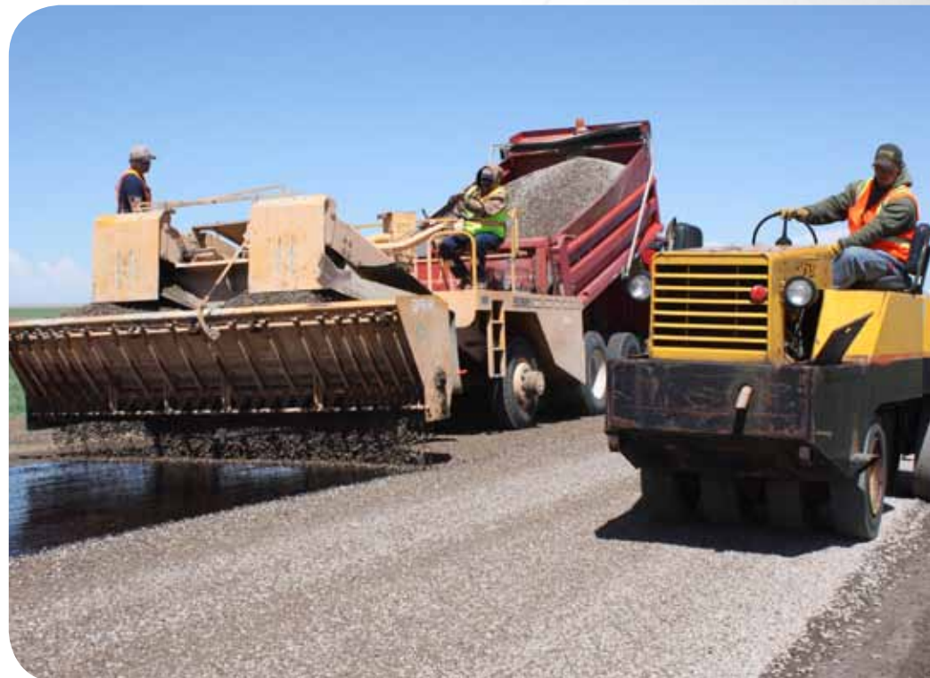
Using its own crews and equipment, Lincoln County Road & Bridge Department applies first course of triple chip seal on reclaimed base.
