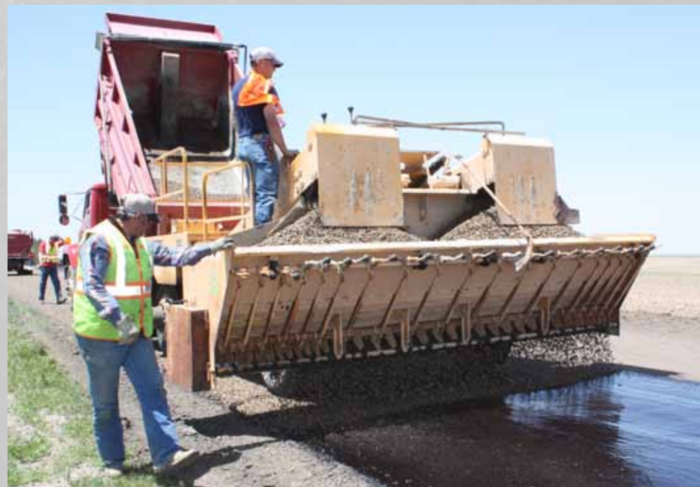
County's Flaherty chip spreader broadcasts 3/4-inch stone at rate between 30 and 35 pounds per square yard for first course.
